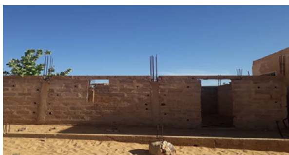
Uncompleted and abandoned classroom built by the project
